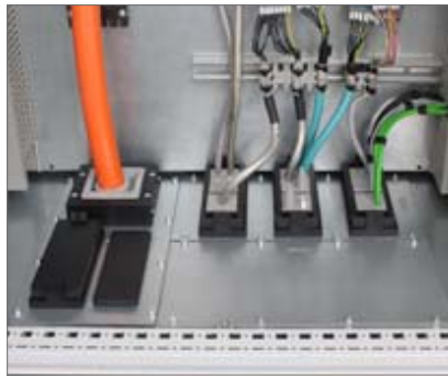
Cable routing via module plates in the base of a Rittal TS 8 enclosure. Mounting with icotek base plate KDR BMP.
